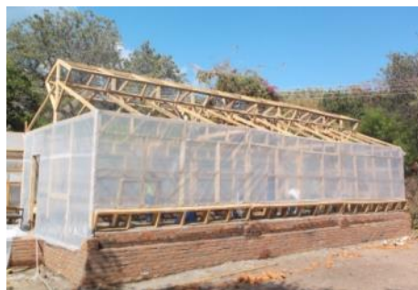
Fasten the polythene sheeting with ripped planks of 0.5" x 2" using 1" wire nails. Cover vents with gauze.
