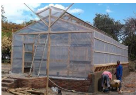
Cover the framework with the polythene sheeting leaving the basal vents open.
