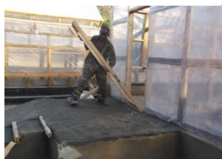
Insert a door made from 2" x 4" planks and covered with chicken wire and polythene.
